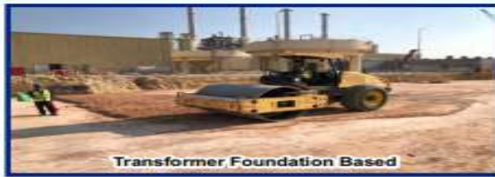
Transformer Foundation Based
