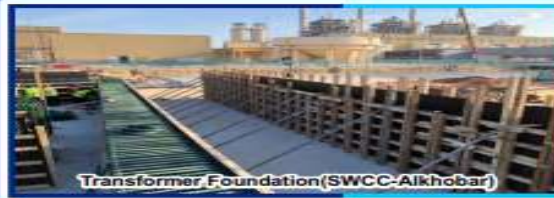
Transformer Foundation (SWCC-Alkhubar)
